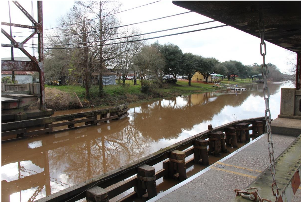
Condition Photo 14: Condition of timber fender system and waterway.
