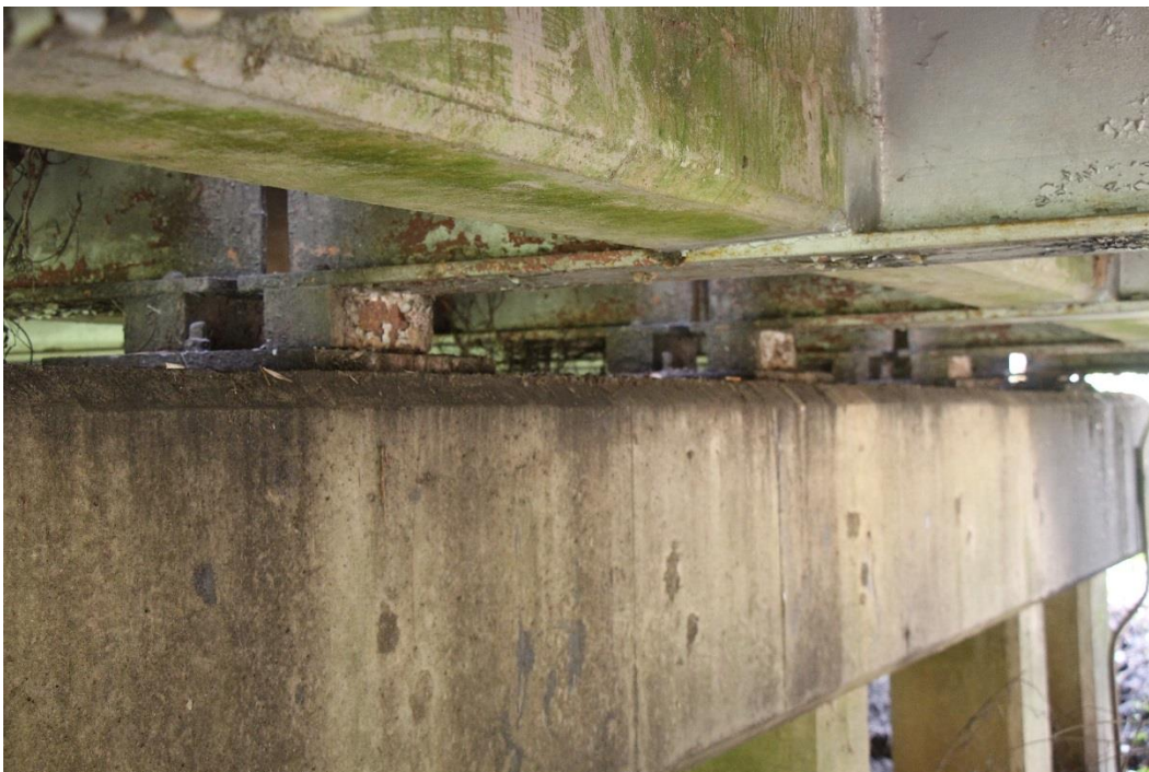
Condition Photo 17: Approach span steel beams bearings, showing corrosion and paint failure.
