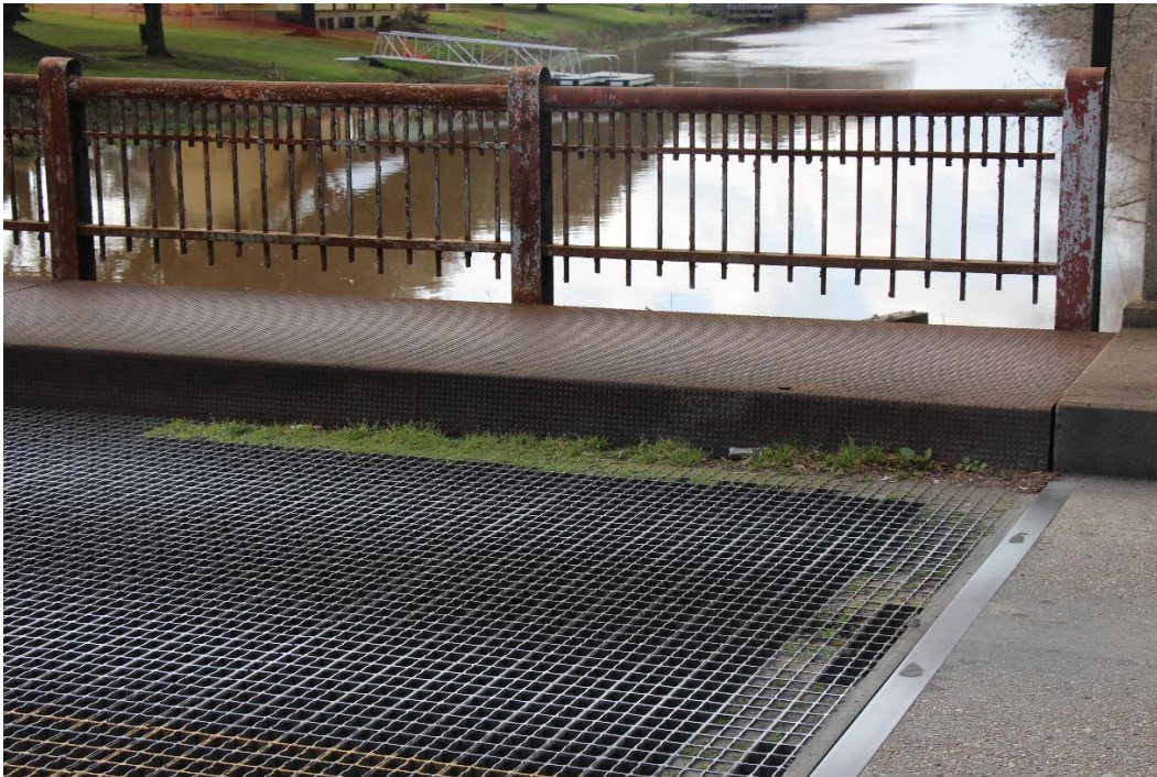
Character-defining Feature Photo 3: Steel grid deck and original metal railings on the vertical lift span.
