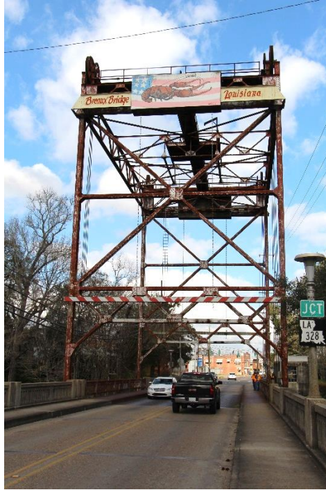
Character-defining Feature Photo 2: Design and construction of a vertical lift span with central drive machinery. The operating machinery, located at the center of a platform, drives the four sheaves on each corner of the lift towers.
