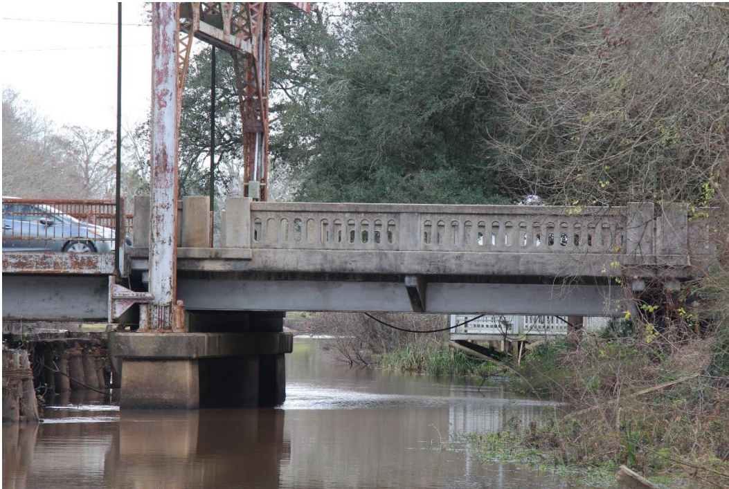
Historic Fabric Photo 1: Typical steel I beam approach span with decorative concrete railing.
