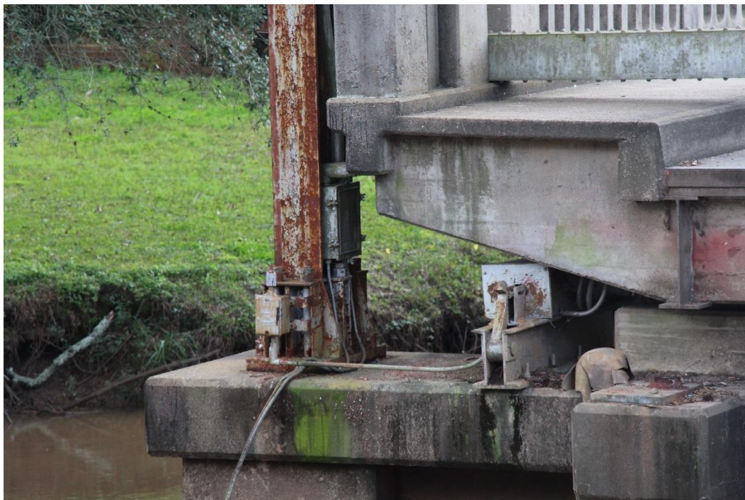
Condition Photo 15: Condition of tower base, span lock, edge of approach span.
