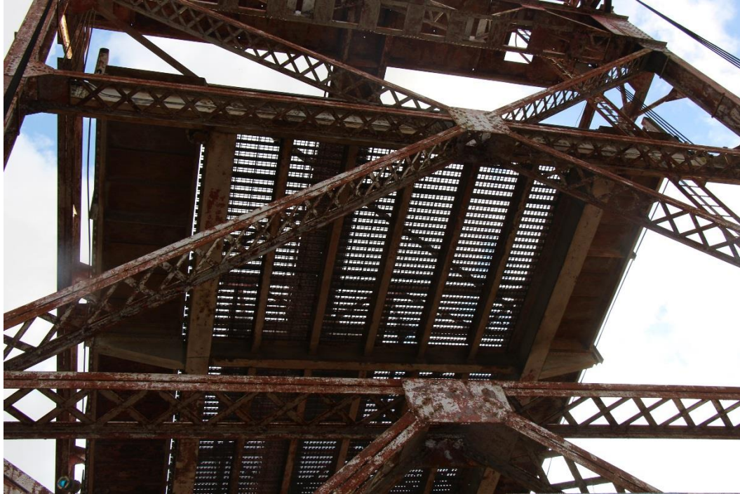
Condition Photo 8: Underside of lift span showing paint failure on all members.
