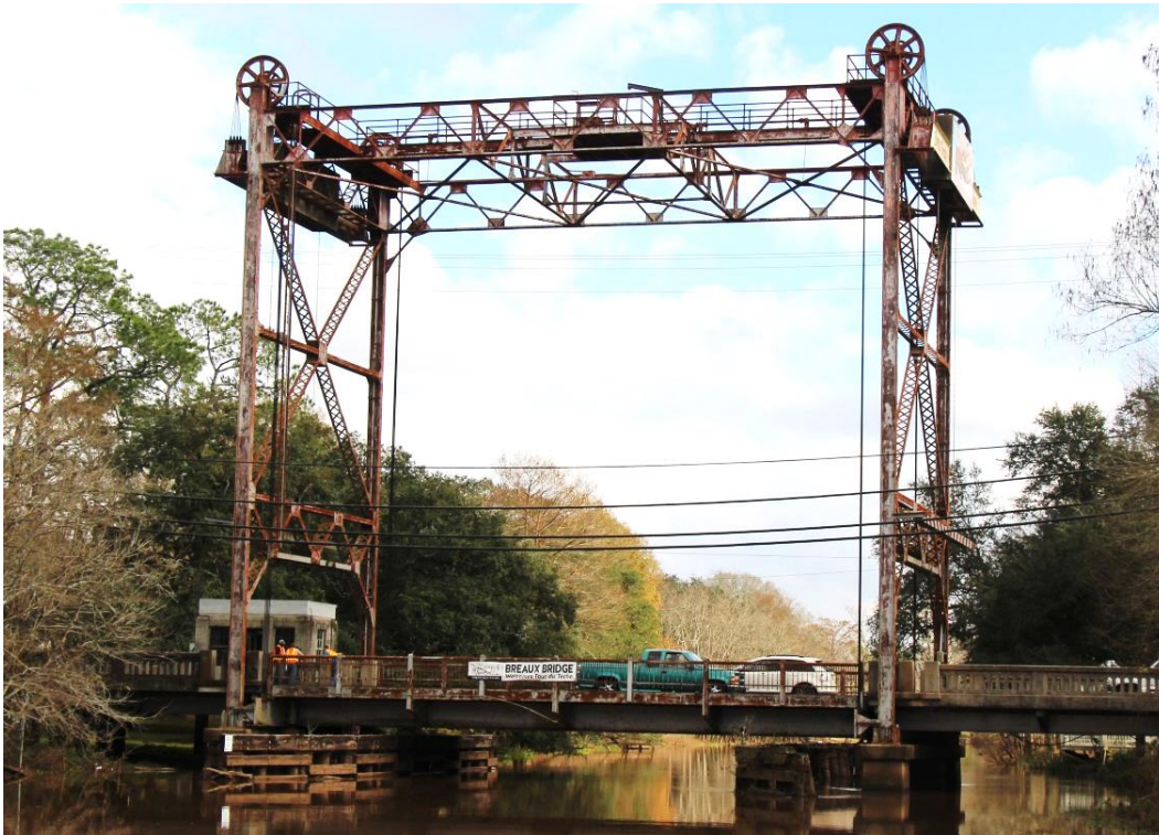
Condition Photo 1: Lift span paint failure throughout.
