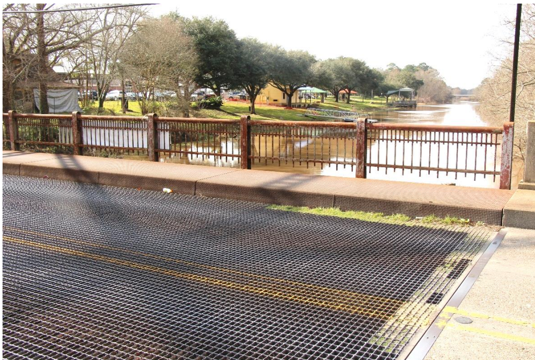
Condition Photo 3: Lift span steel grid deck, metal plate sidewalk, metal railing.
