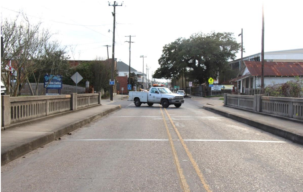
Condition Photo 10: Concrete deck of west approach spans; note truck used to block traffic.
