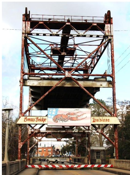
Condition Photo 5: Lift span partially open, condition of structural steel, paint failure.
