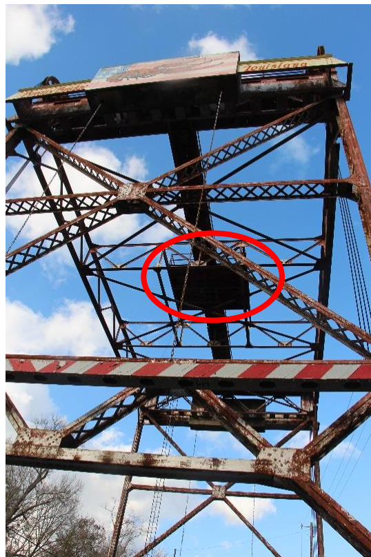
Condition Photo 9: Machinery platform in middle of lift span; traffic barrier gate condition.
