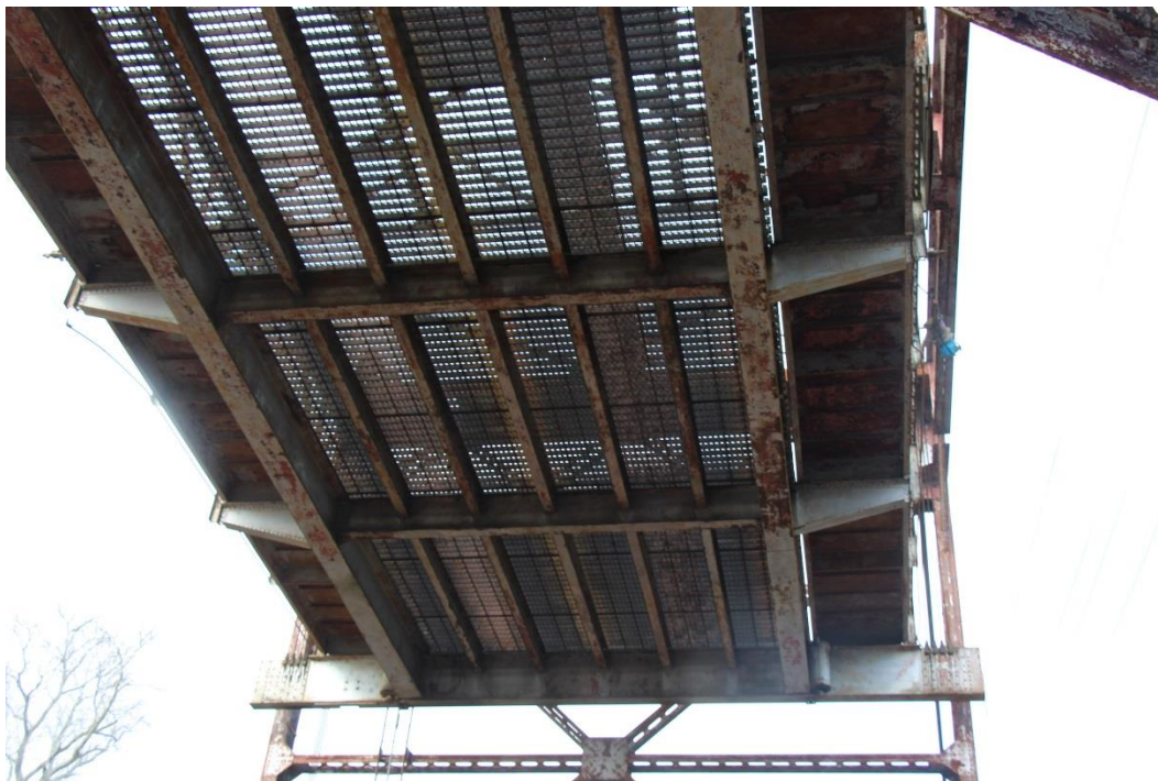
Condition Photo 7: Underside of lift span showing paint failure on all steel members.
