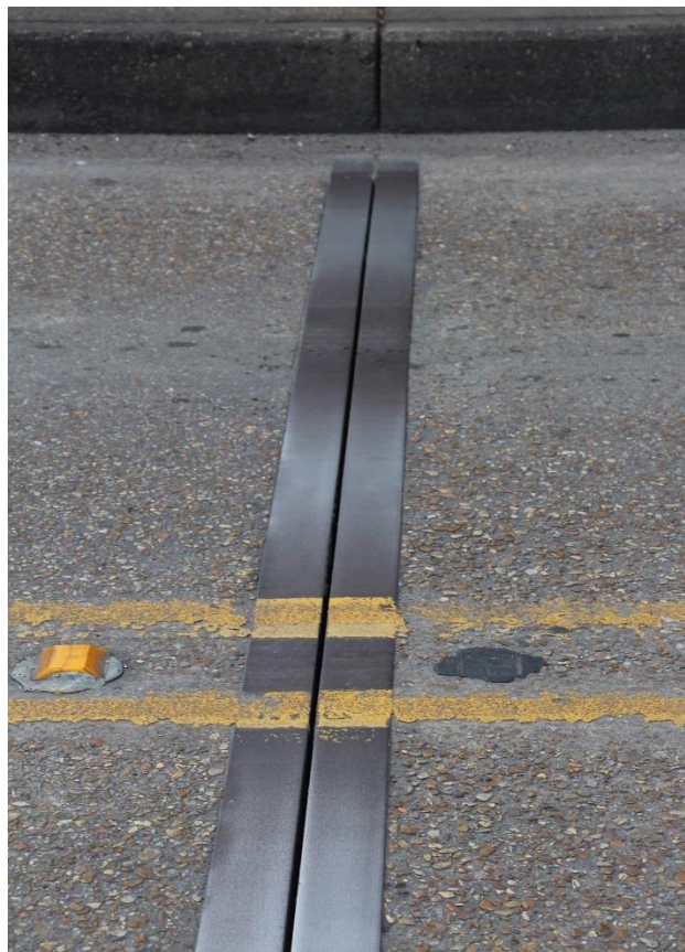
Condition Photo 11: Typical expansion joint in roadway deck of approach spans. Note that the joint is not sealed and there is scaling on each side of the steel armor members.
