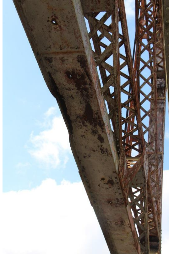
Condition Photo 16: Impact damage to bottom horizontal member of end portal in tower.
