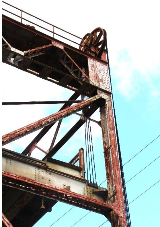
Condition Photo 6: Machinery and cables atop tower, counterweight paint failure.
